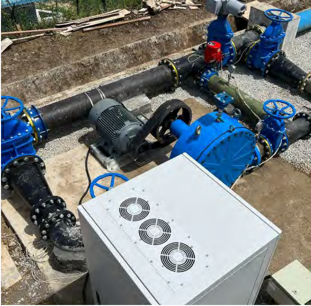
Figure 1: The Super Butterfly In-Pipe Hydropower System.
