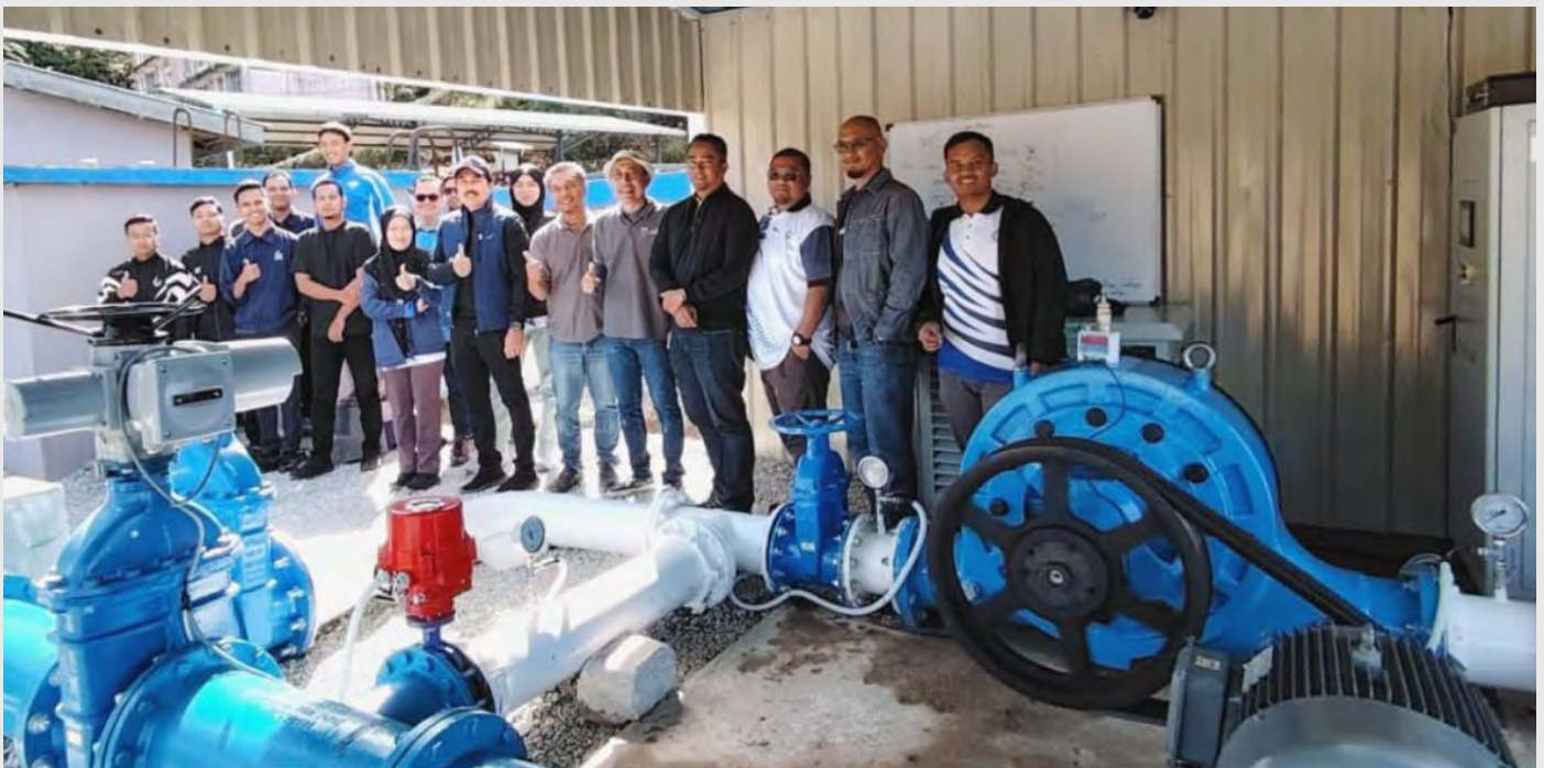
Figure 2: Operational pilot installation of the Super Butterfly In-Pipe Hydropower System at Brinchang, Cameron Highlands.
